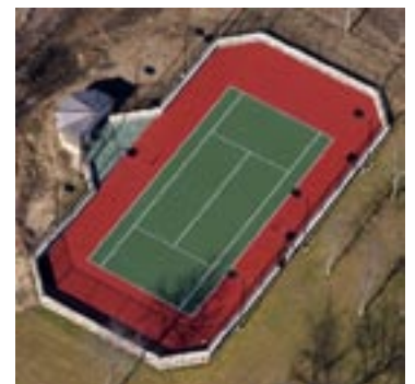
Four coats of cushion and a red and green acrylic court color were installed over the concrete.
